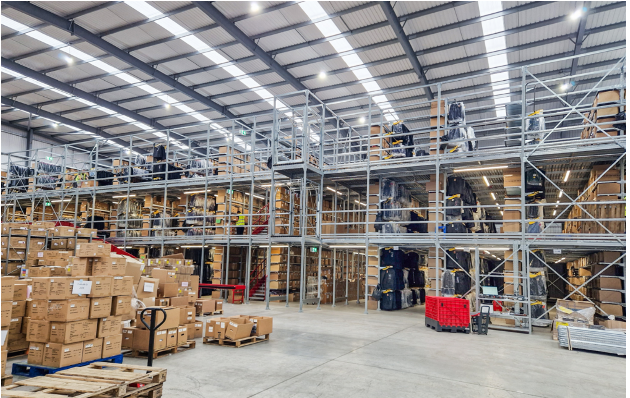
Super 4-5-6 Fashion Multi-Level Warehouse Reference Installation <August 2024>
